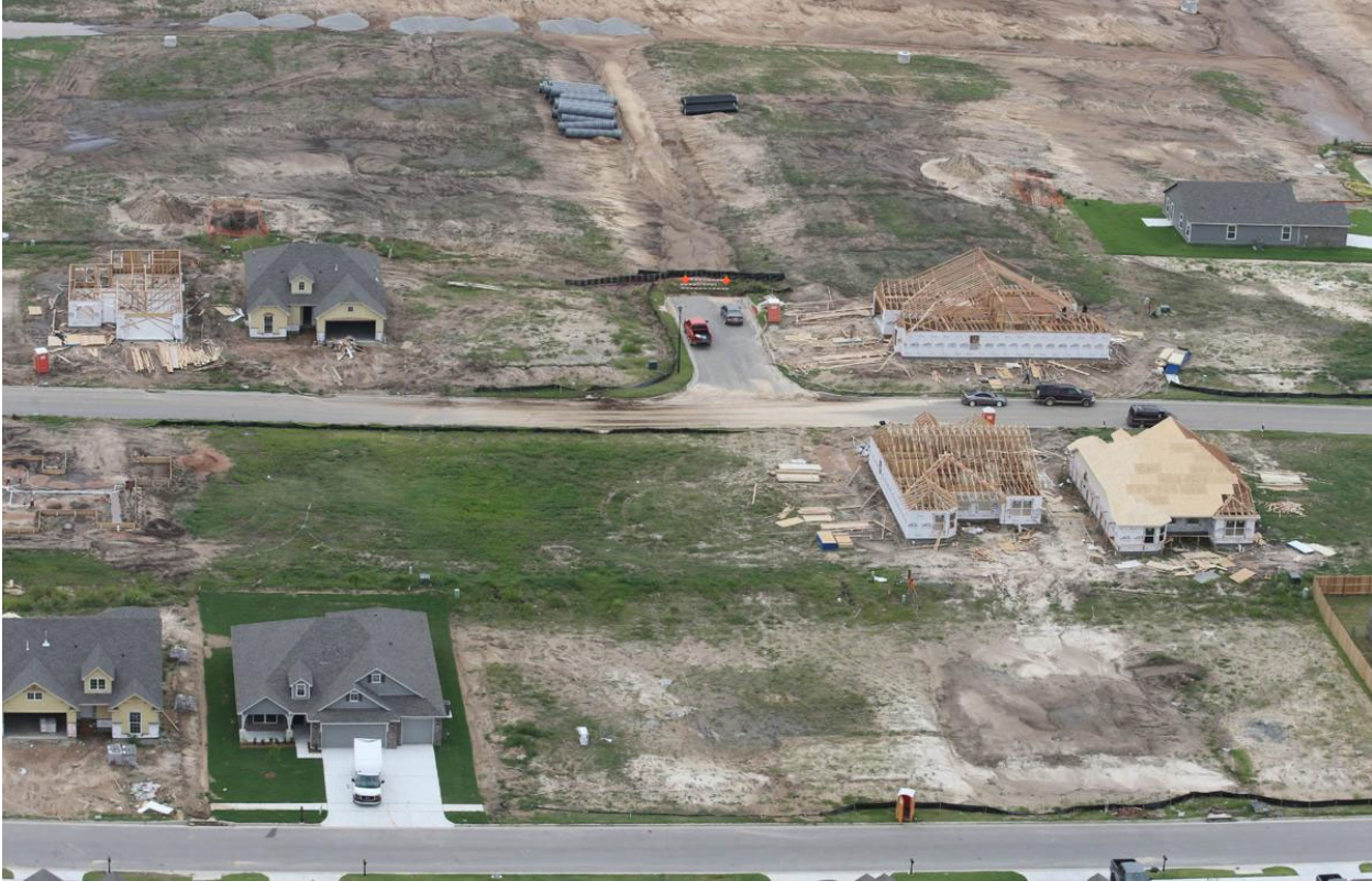
Homes are pictured under construction in the Tulsa area. The number of housing starts in the city is on pace to set a record this year. Tulsa World file
